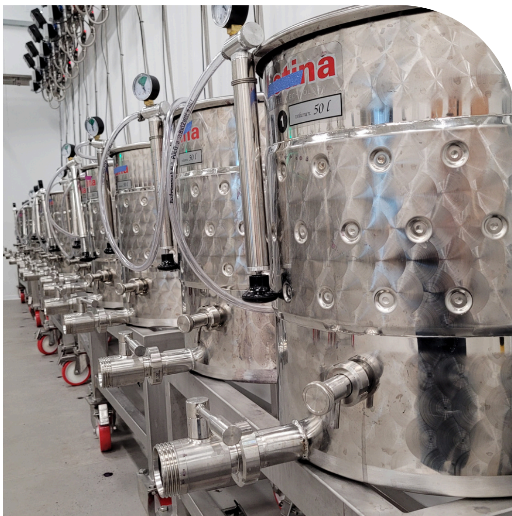
Research tanks at Niab's Wine Innovation Centre, East Malling
